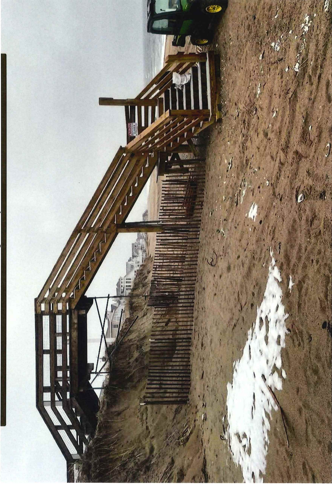
Beach Access 8 Current Conditions. 4 Helical Piles to be replaced by others.
