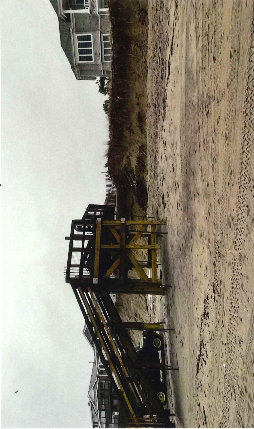
Beach Access 10 Current Conditions. Boardwalk to be Removed to be by others 02/01/24
