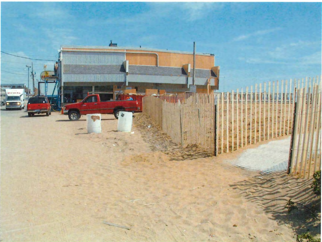
PHOTOGRAPH 16: THE COMPLETED DUNE AT THE END OF BROADWAY ST. WITH SNOW FENCE AND MOBI-MAT.
