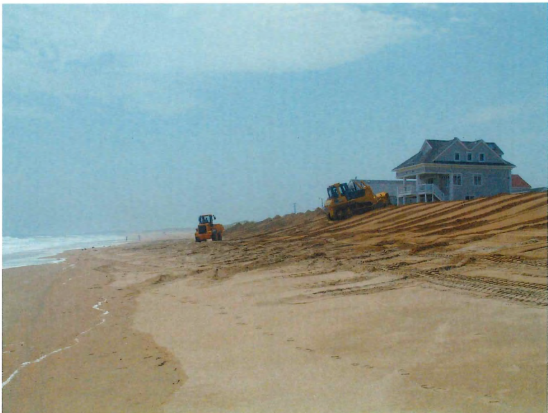
PHOTOGRAPH 16: LOOKING SOUTH AT THE PILES TO BE FORMED INTO THE PROPOSED DUNE.
