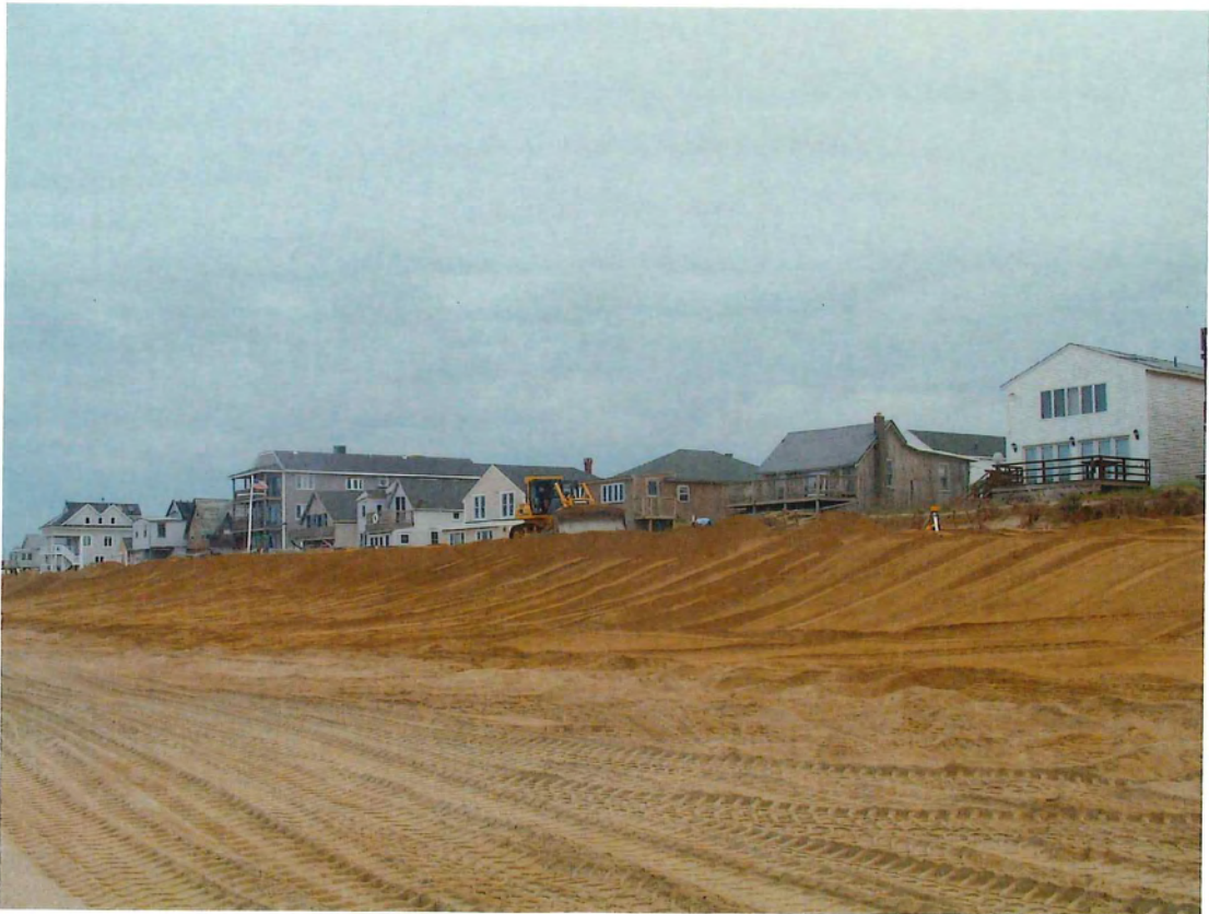
PHOTOGRAPH 8: BULLDOZER SHAPING THE NEW DUNE AT THE ATLANTIC AVE. SITE LOOKING SOUTH.
