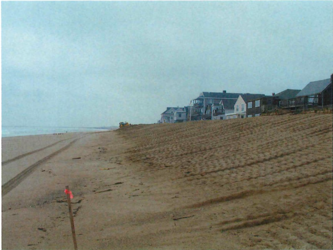
PHOTOGRAPH 13: A VIEW OF THE COMPLETED HALF OF THE PROPOSED DUNE LOOKING SOUTH.
