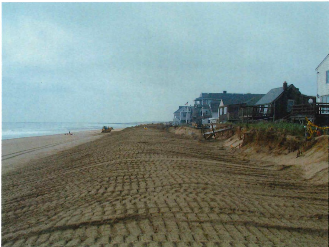
PHOTOGRAPH 14: A VIEW FROM ATOP THE COMPLETED HALF OF THE PROPOSED DUNE LOOKING SOUTH.
