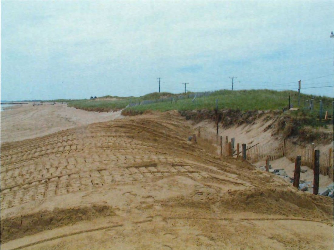
PHOTOGRAPH 10: SOUTHERN END AND TRANSITION NEEDS TO BE FINISH GRADED.
