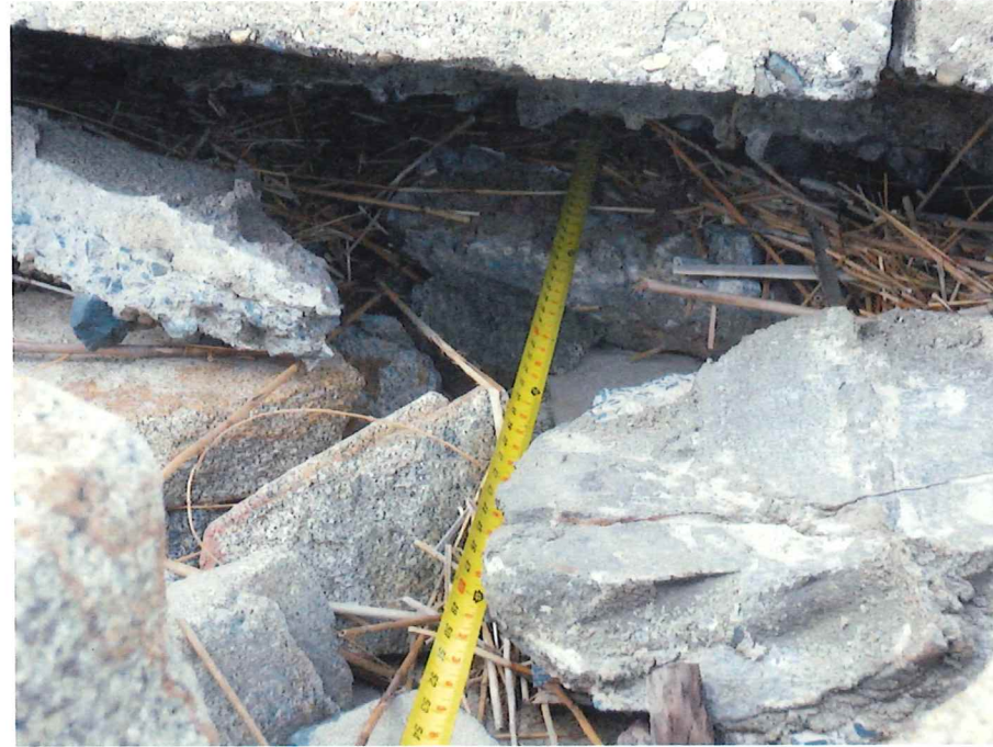
PHOTOGRAPH 3 Void between concrete seawall and stone mound.
