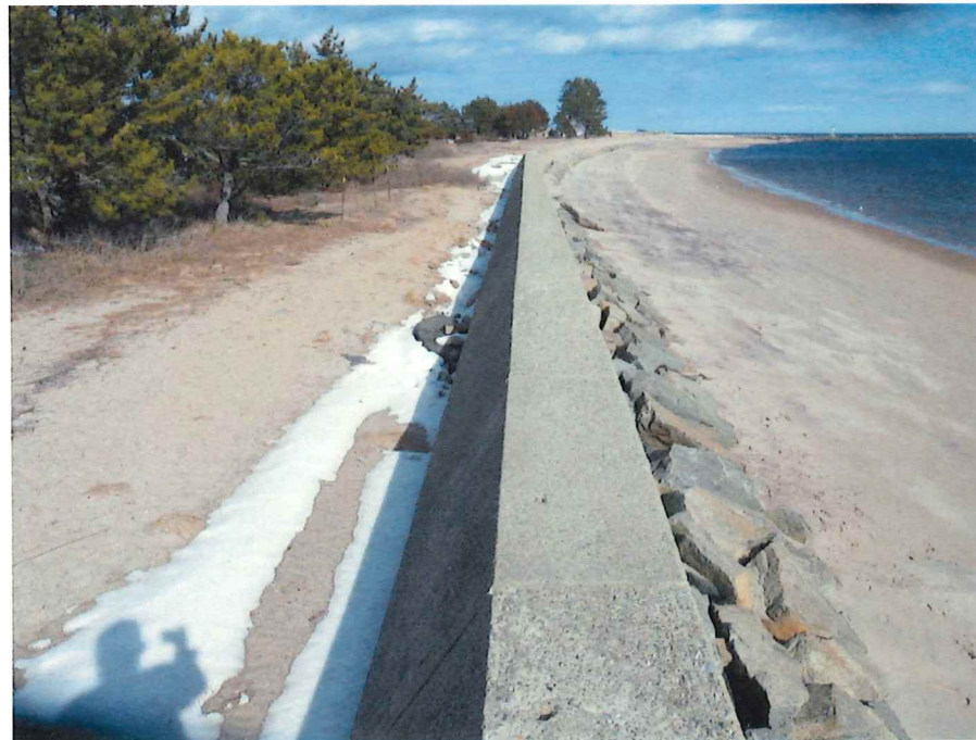
PHOTOGRAPH 4 Sinkholes along landside of seawall.
