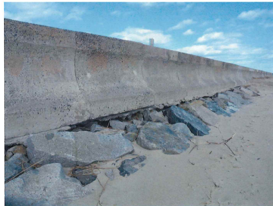
PHOTOGRAPH 2 Typical photograph of concrete seawall and stone mound (Note: voids between stone mound and concrete leveling course)
