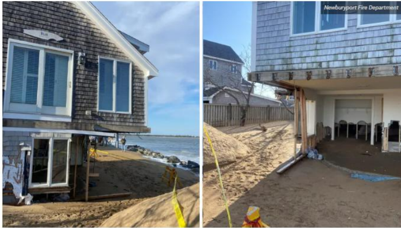
A damaged vacant home on Massachusetts' Plum Island after a storm blew through on Friday, Dec. 23, 2022.
